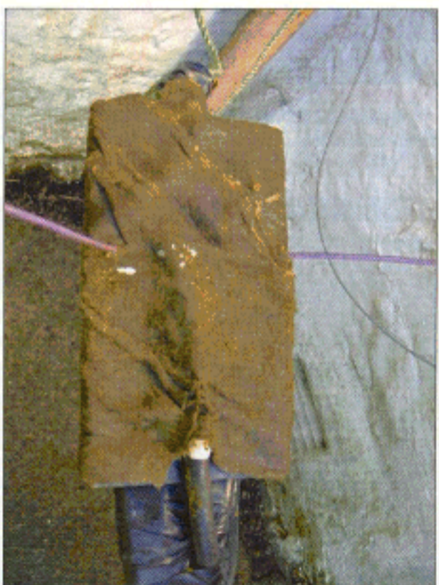
Fig. 5: Waterproofing the centre-piece with sticky Denso Tape keeps the weather out of the joints.
